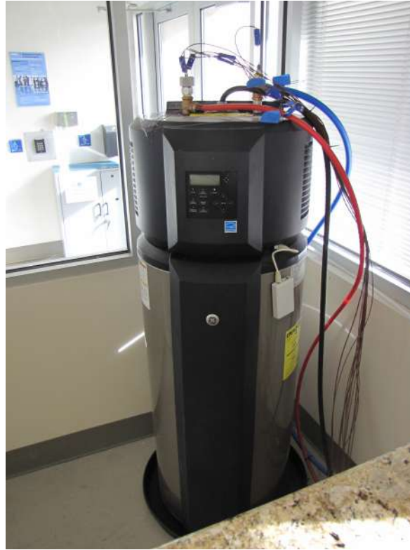
Figure 3. Residential water heaters are a flexible load that can provide a range of grid services—including load shifting and frequency regulation—without impacting occupants. This GE heat pump water heater is shown being tested at NREL’s Advanced Home Energy Management Laboratory. Image courtesy of NREL.
